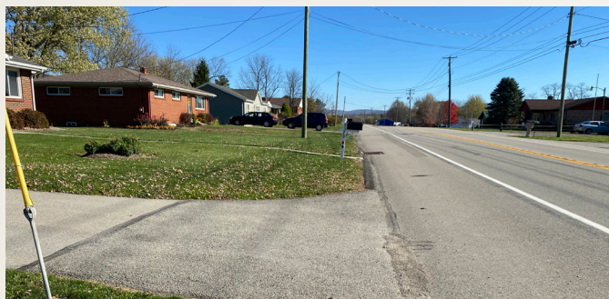
Driveway tie ins will be incorporated into the new alignment. (SR 981, V10 Project at Arnold Palmer Regional Airport)
